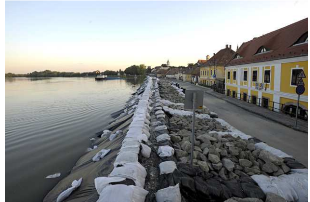
Pic. 15: Heightening with rip-rap-reinforced sandbag wall at Szentendre before the flood - 2010
