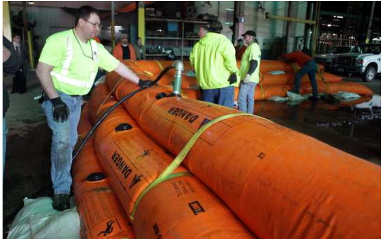
Pic. 23: A 3 tube high system under filling
