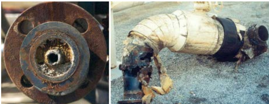
Fig. 24: Scaling and corrosion in a geothermal pipes (picture: NREL, Keith Gawlik)
