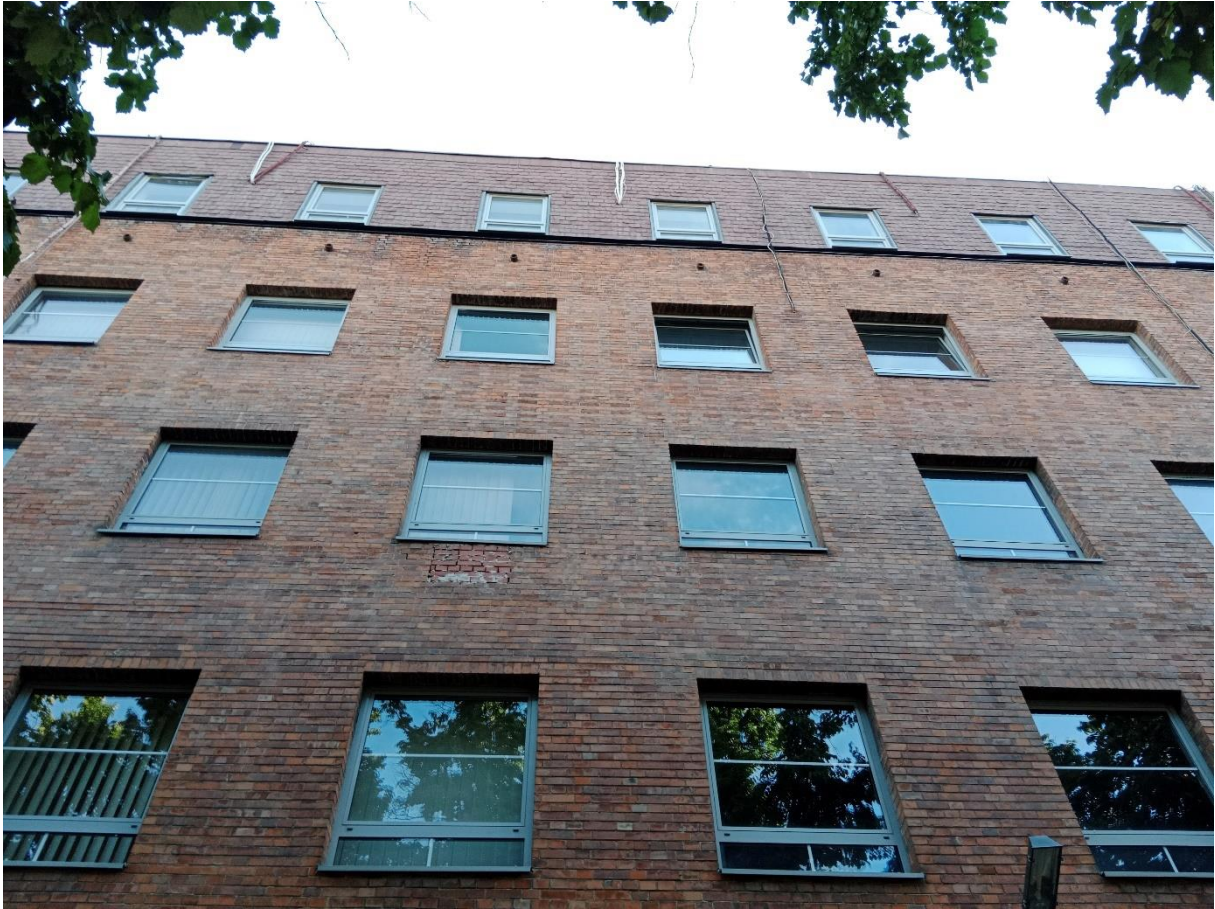
Figure 11 Facade with marks of former intervention
