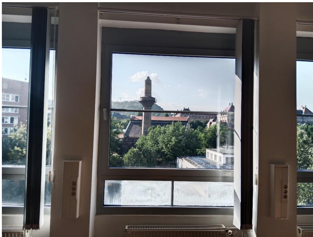
Figure 10 Window with moisture
