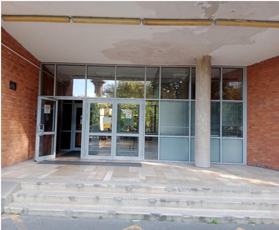
Figure 9 The main entrance with wet marks
