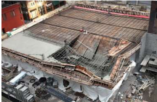
Figure 5. Wooden Formwork Failure in Construction (source: Civil Engineering Forum [33])
