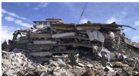
Figure 1. Damaged building after the 6 February 2023 Türkiye-Syria Earthquake (source: Magdalene College – University of Cambridge [6])
