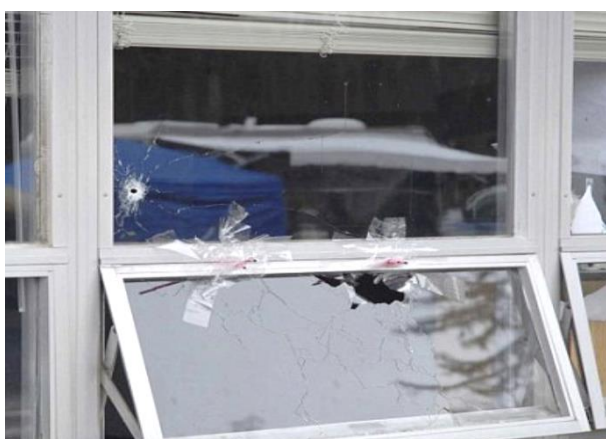
Figure A8. Penetrated Window of Classroom 10 at Sandy Hook Elementary School (Bates)
