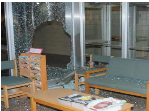
Figure A4. Destroyed Pane-Glass Window Inside Sandy Hook Elementary School (Appendix to Report A171)
