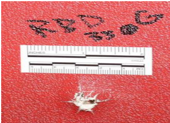
Figure C6. Penetrated Interior Wall of Classroom 109 (Cardenas, Natalie, et al.)
