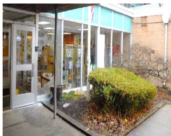
Figure A3. Destroyed Pane-Glass Window Outside Sandy Hook Elementary School ( Appendix to Report A167 )
