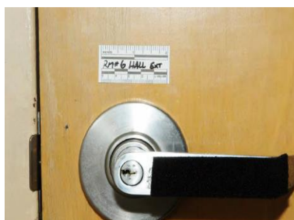
Figure A7. Interior Door Lock (Hallway Side) (Appendix to Report A178)
