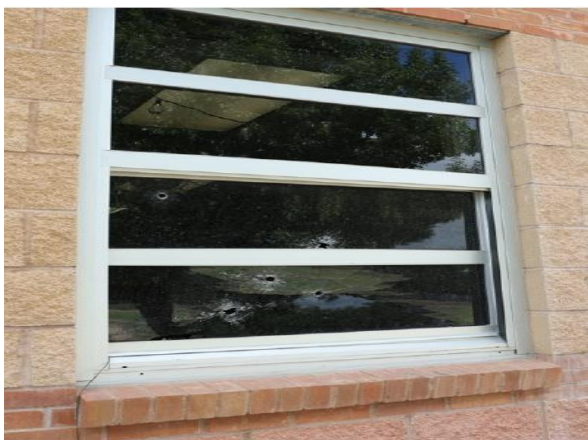
Figure C8. Penetrated Classroom Window of the West Building at Robb Elementary School (ALERRT 12)
