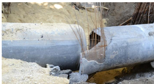
Fig. 1 The failure of Sentab type water pipe in 2012
