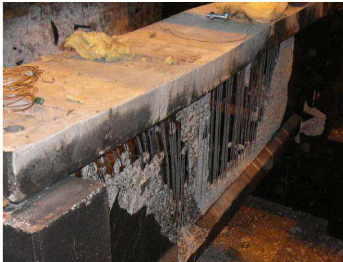
Figure 4: Beam with the reference concrete (Mix A) after failure in 12 minutes
