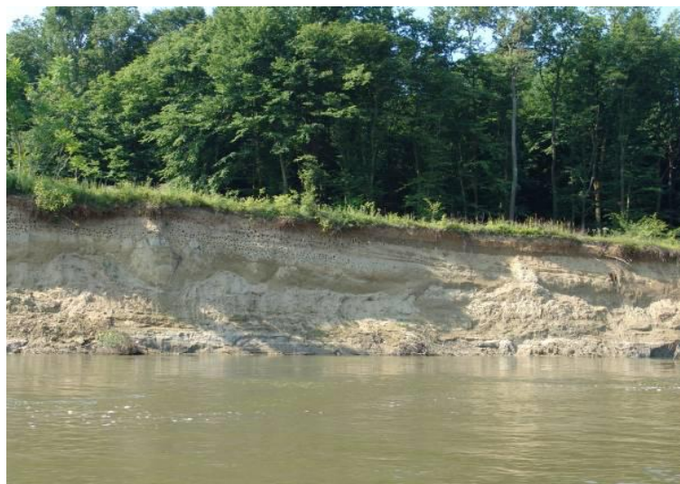
High bank exposed to intensive erosion, 61+500 km
