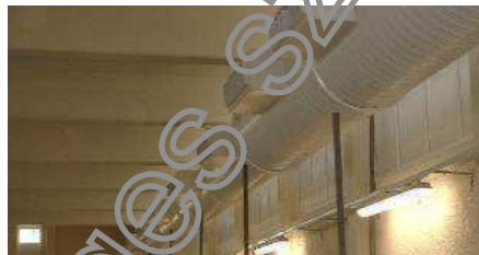
Fig. 3. Air duct with grills, case A
