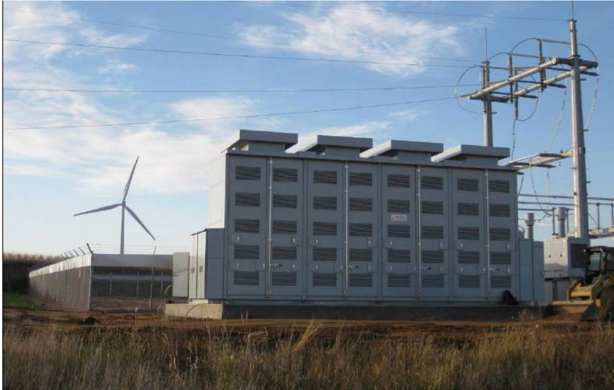
14. Figure: XCELL batteries supporting wind turbines (USA) [2]
