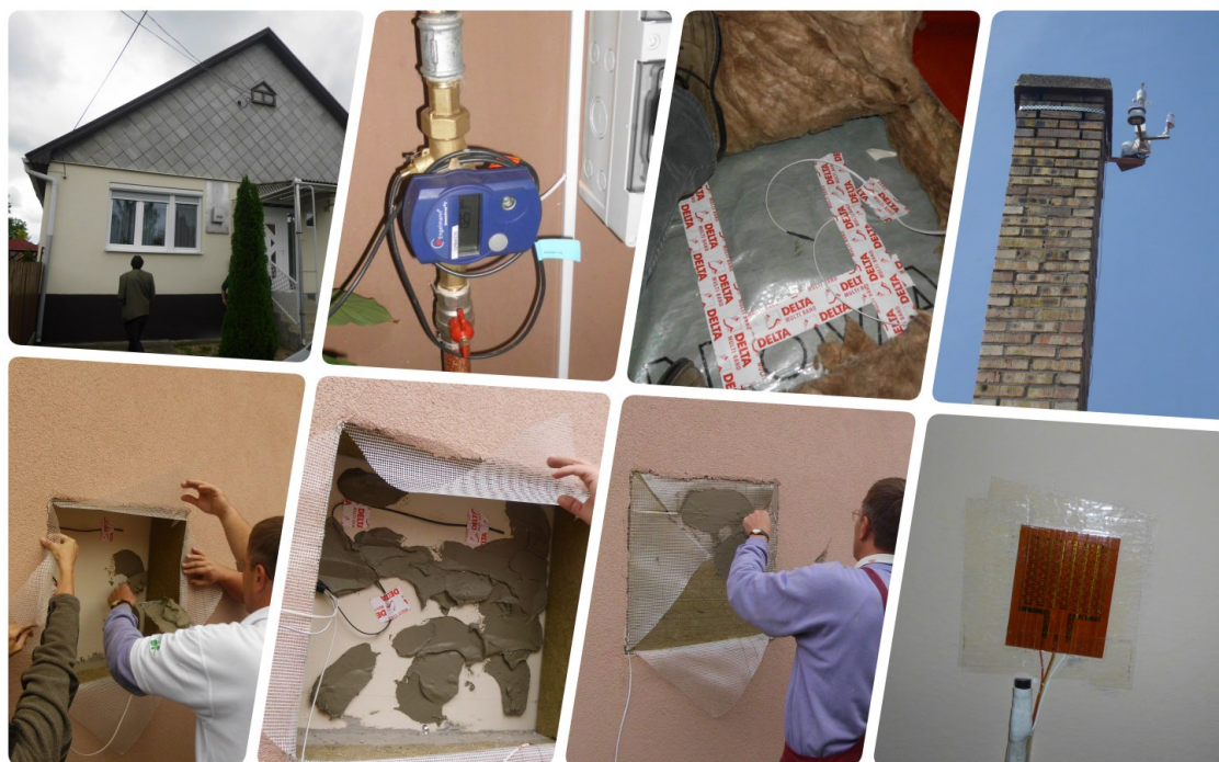
Fig. 1 From top left to bottom right: house in Hajdúnánás before the insulation process; thermal energy meter built into the heating system; sensors in the attic; weather station on an unused chimney; sensor installation on the façade; heat flux meter on the inner wall
