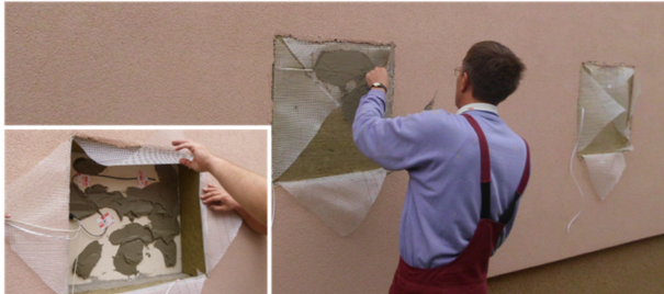
Figure 3: monitoring sensor installation in the wall with different ETICS installation technique
