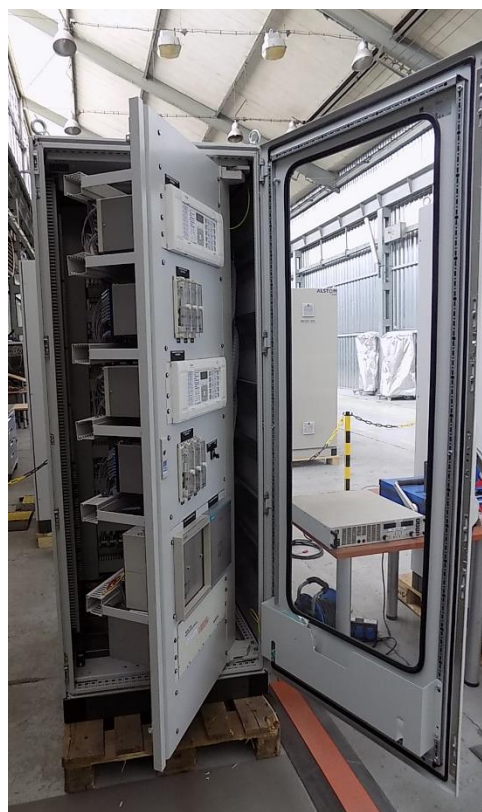
Fig. 1. Existing generator protection panel.
