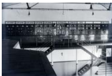
Figure 7. Switch room of power plant Ikervár (Fortepan 1928)
